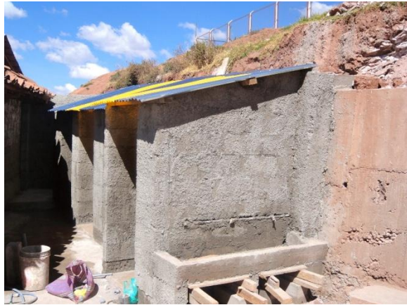
June 2012 – Work in progress! Eliza from GVN Foundation visits to check how everything is going.
